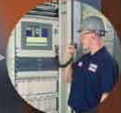
Public Address/ General Alarm
