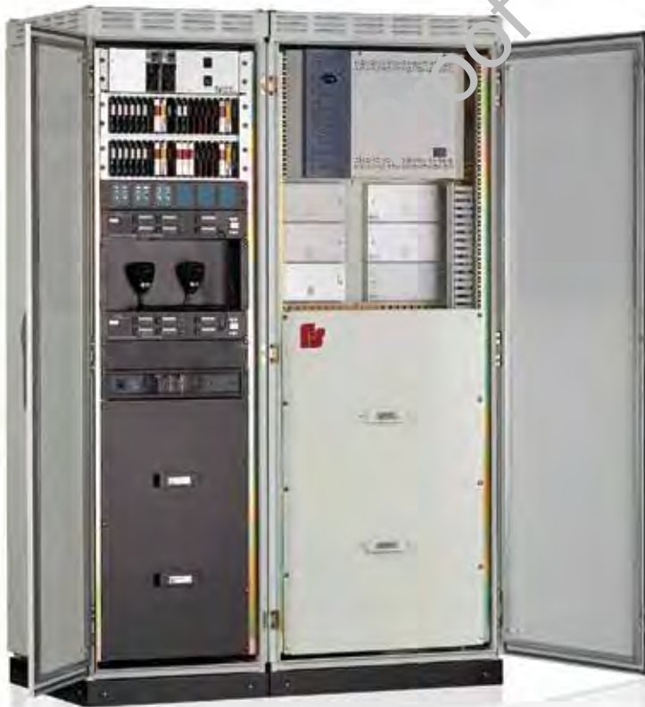
Rack mounted Echo System
